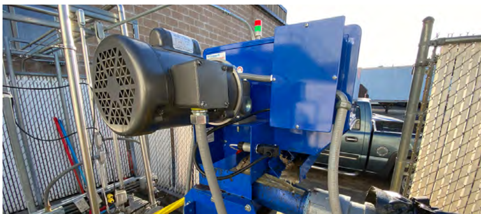
Water skimmer at the Bridgeton, Missouri plant
