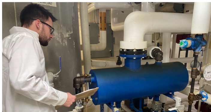
High-efficient condensate pump at the Covington, Virginia site
