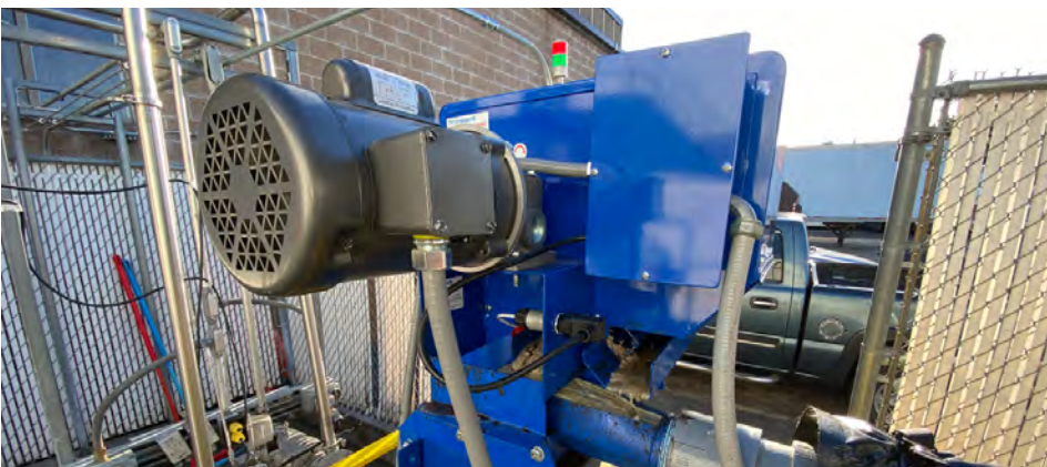
Water skimmer at the Bridgeton, Missouri plant
