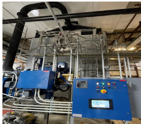
The new boiler at the Verona, Missouri site
